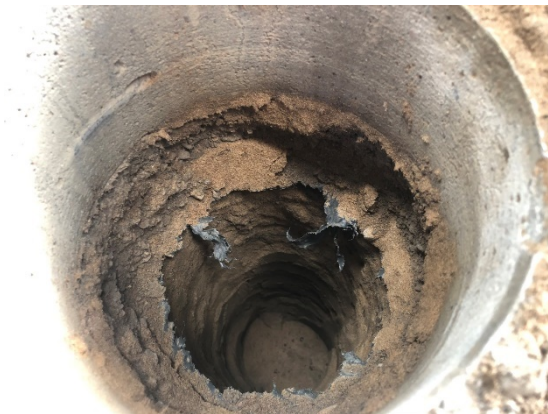
Photograph 3: Illustrative concrete thickness and underlying soil.
